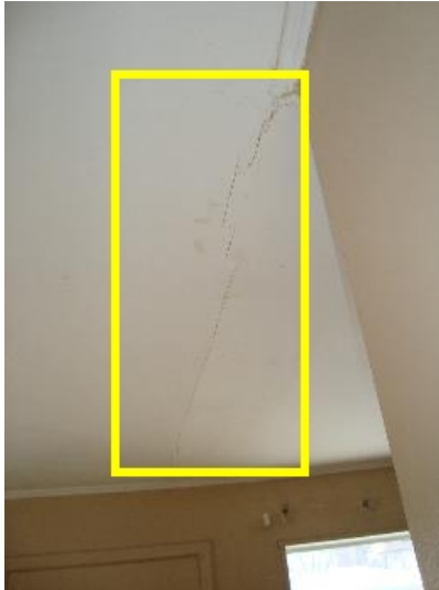
hairline crack runs from wall to wall
