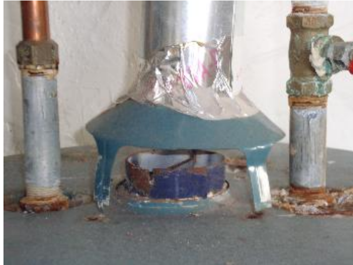
rust and faulty hood connection
